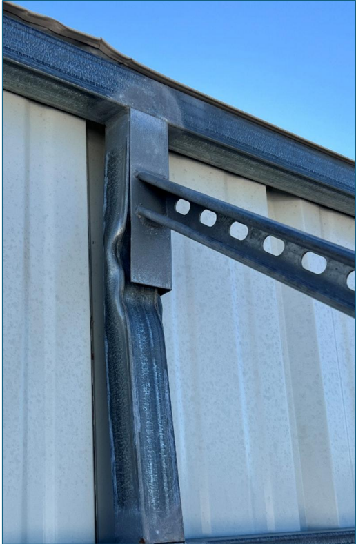
Photos of Linea Screen damage
